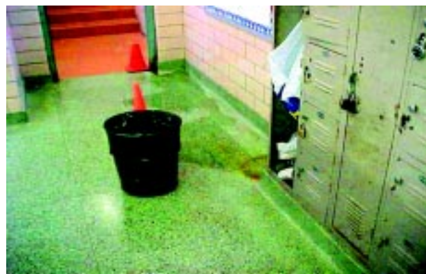
Clean up water to prevent mold growth.
